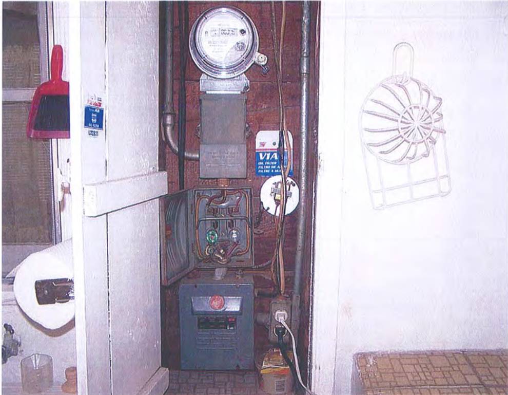
Smart Meter on porch
